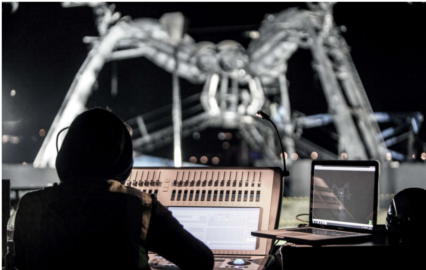
Below: An Avolites Sapphire Touch console provided lighting control and triggered flames, pyrotechnics and lasers with on-site support from the Avolites team.
